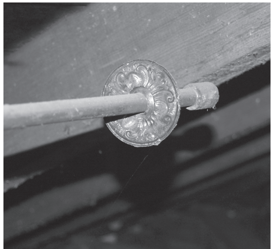
Capped-off gas pipe with original escutcheon.
