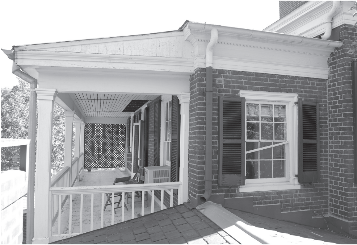
Southwest corner of rear addition. The bottom rail of the upper window sash on the south elevation has failed. A heavy application of sealant has been applied above the step flashing and between the dissimilar metals of the step flashing and ridge. Brick replacement and pointing repairs have not been carefully executed.
