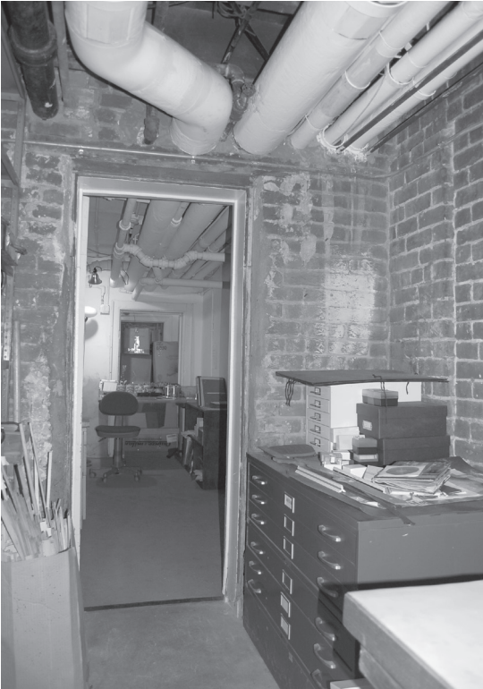
Room B11, looking north. The integrity of the brick basement walls has been compromised by the piping required for the central grounds heating system.
