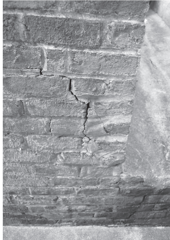
The brick masonry of the retaining wall at the east end of the areaway is cracked and displaced.
