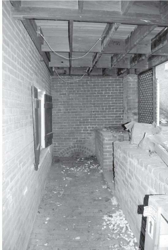
Basement areaway along the west elevation, looking south; note the arch for the drain at the base of the south wall
