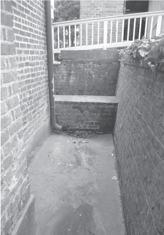
The north areaway is wet and supports the growth of algae, moss, and lichen. The drain grate is corroded and clogged with leaves.
