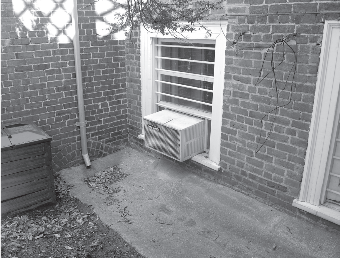
Arch for drain at the base of the southwest addition's east elevation
