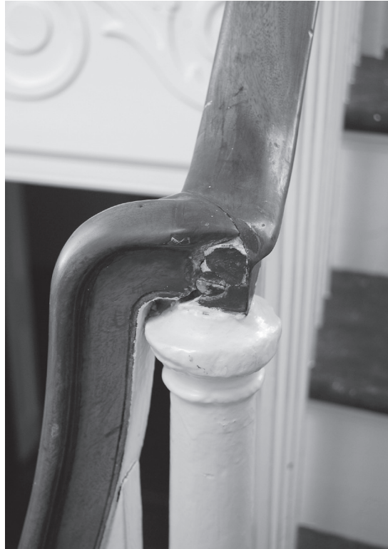
The mitered joints of the handrail on the stairway have been poorly repaired and infused with fillers.
