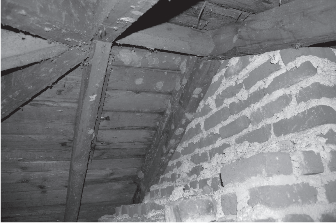
View of the rafters and ridge beam. Note the ledgers (fastened to the two rafters immediately south of the chimney breast) that may be evidence of an early roof hatch.
