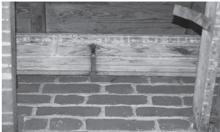
Removal of the second-story ceiling from room 207 revealed the original west entablature with its original paint
