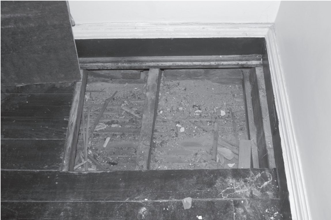
A probe in March 2010 revealed the possible location of a dumbwaiter in room 107
